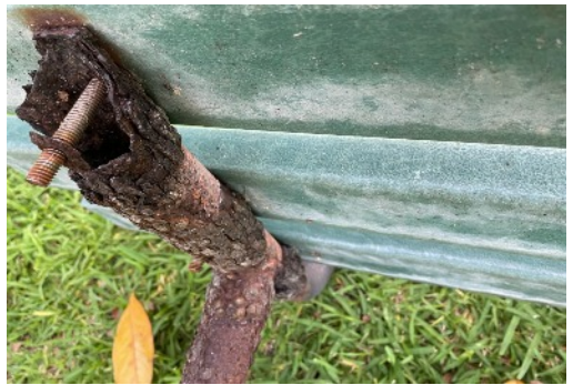
Rusted bench frame
