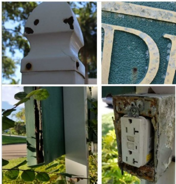
Showing deteriorated sign and electrical outlet
