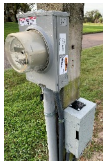
New meter and electric panel
